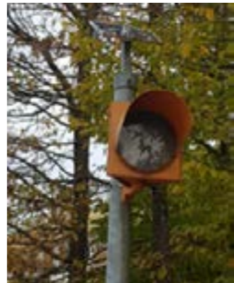
Figure 2.4 Traffic Light with solar panel at Gökçöy
