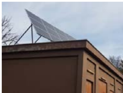
Figure 2.5 Roof Mounted Solar Panels at Gökçöy Campus
