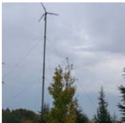
Figure 2.6 Wind Turbine at Gökçöy Campus
